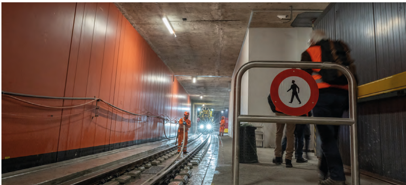
Hosing down the concrete dust during construction in the Forch tunnel. Photo Peter Hefti.
